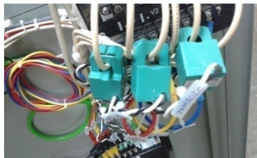
Clamp on type current transformers installed on the secondary side
